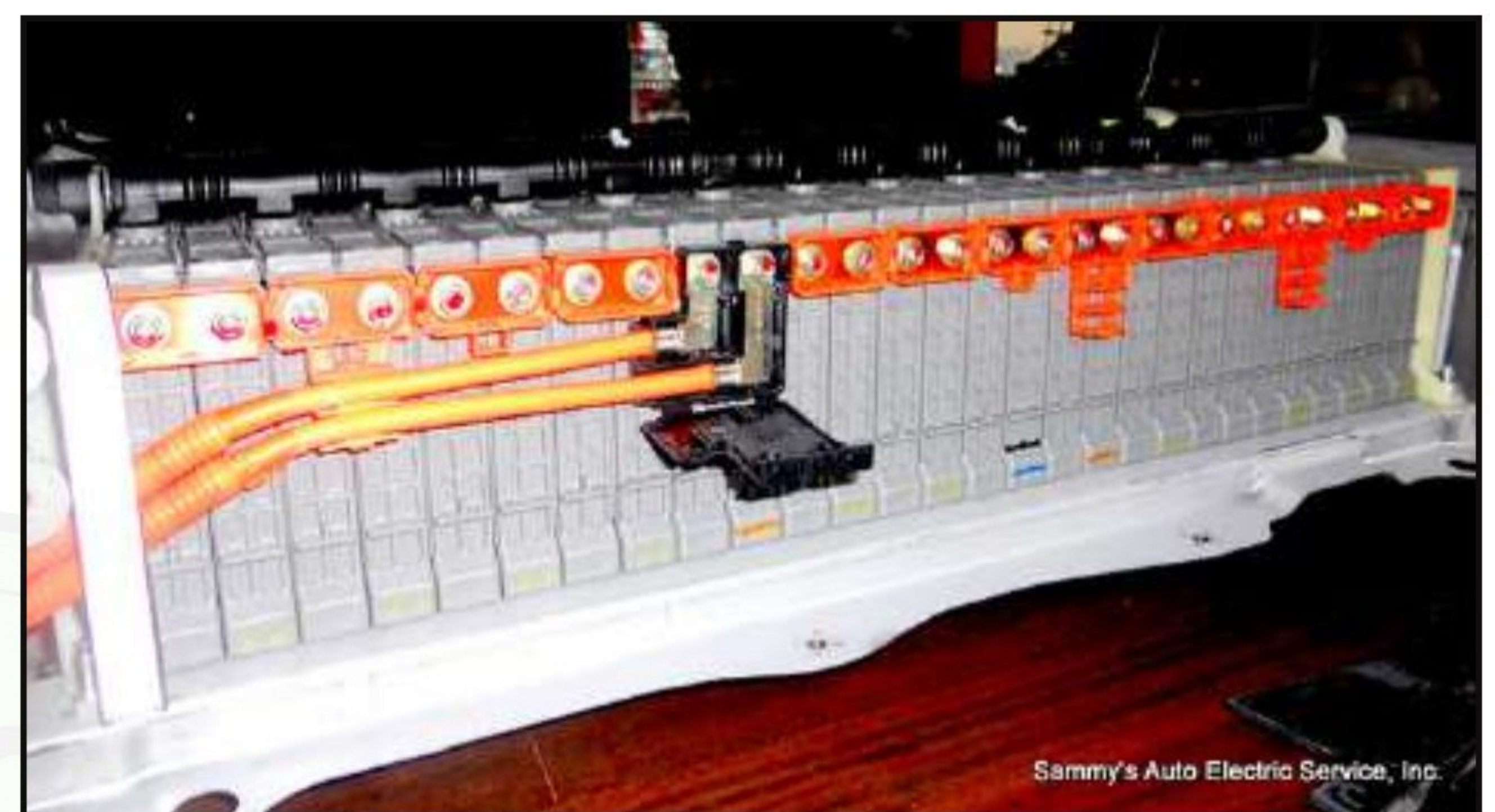
Figure 9 – Service Plug Split between Modules 19-20 (Battery Block#10)
