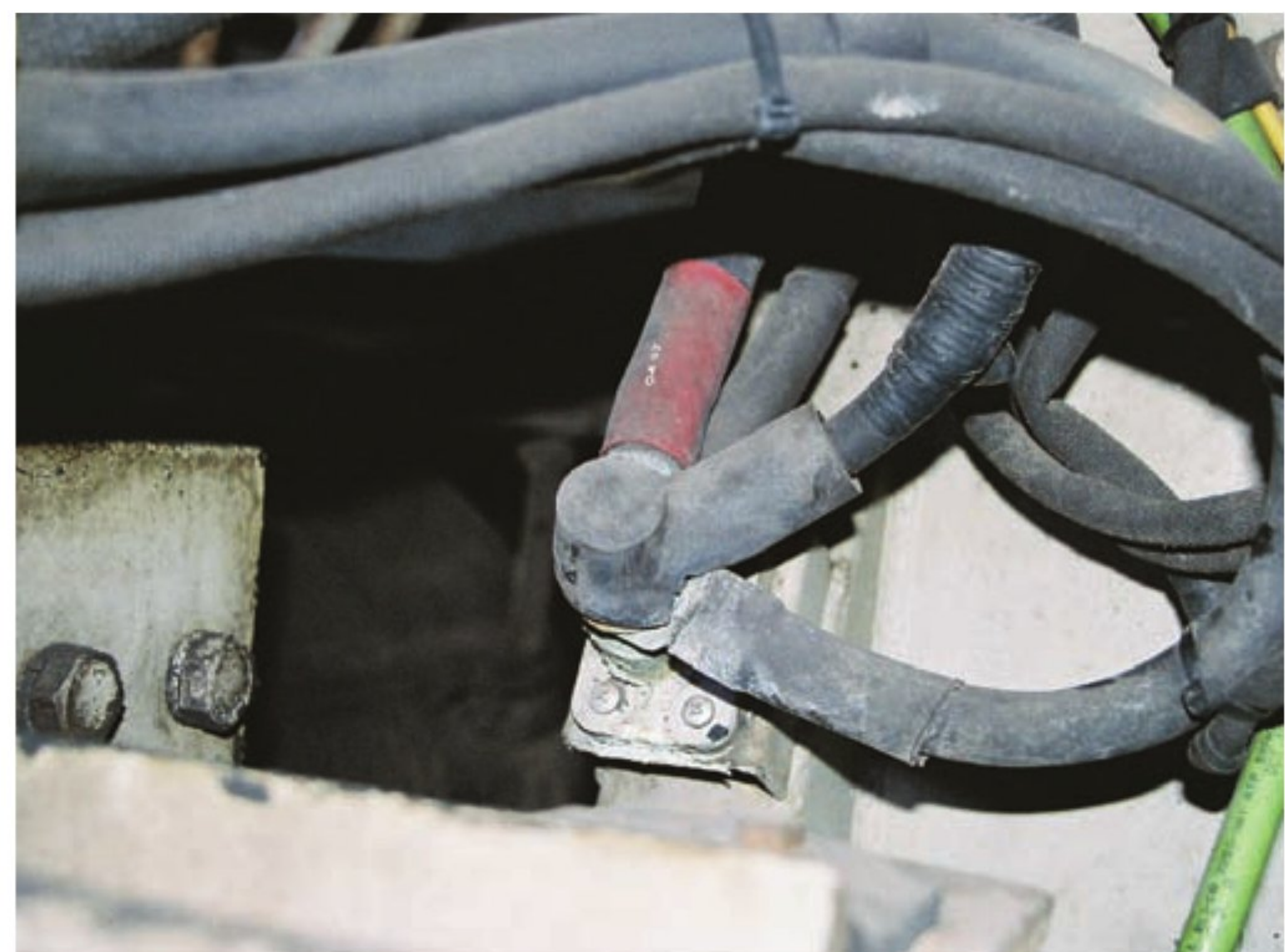
Photo 8A: Bulkhead Connection 50-DN
